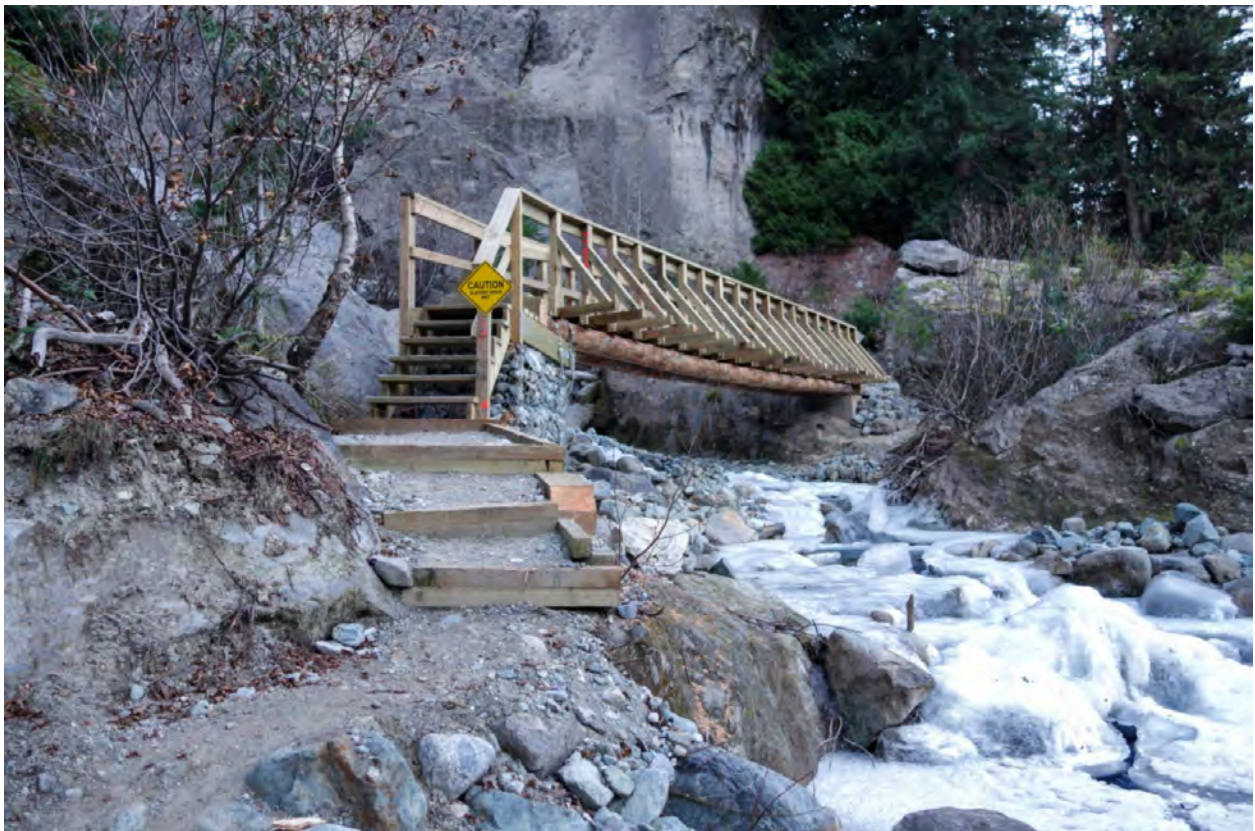
Photo 8. The Truckwash Creek footbridge. The bridge may be destroyed by debris flow activity. Further small, Class 1 snow avalanche from the left ravine sidewall may affect the crossing site and damage the bridge.
