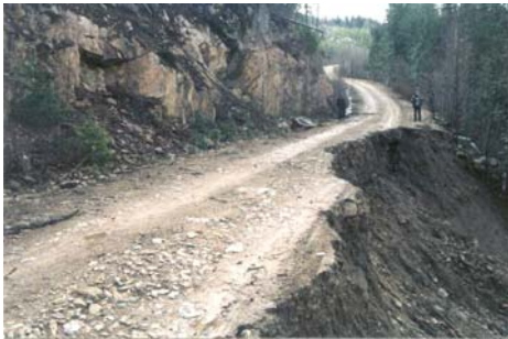
Influence of an excessive amount of water on road stability. (Photo: Tim Giles)
