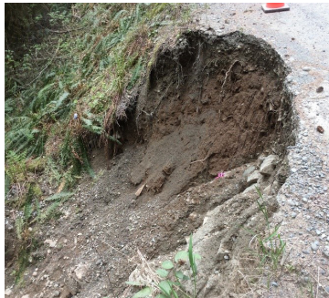
Blocked culvert and road destruction
