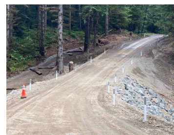
Reflective steel posts to delineate the road
