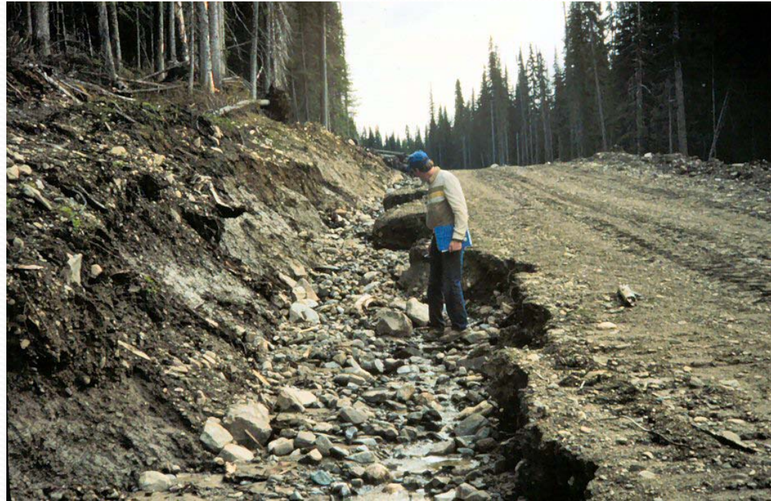
Insufficient cross-drainage resulted in the capture and routing of water along road ditches. (Photo: J. Schwab) Source: Pike et al. 2010.
