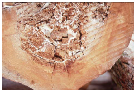
Brown crumbly rot decay with white mycelium.
