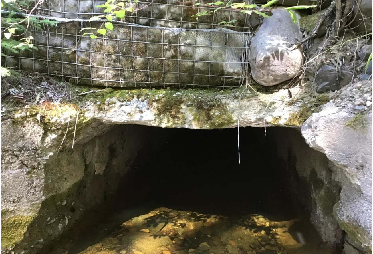
Headwall degradation at outlet
