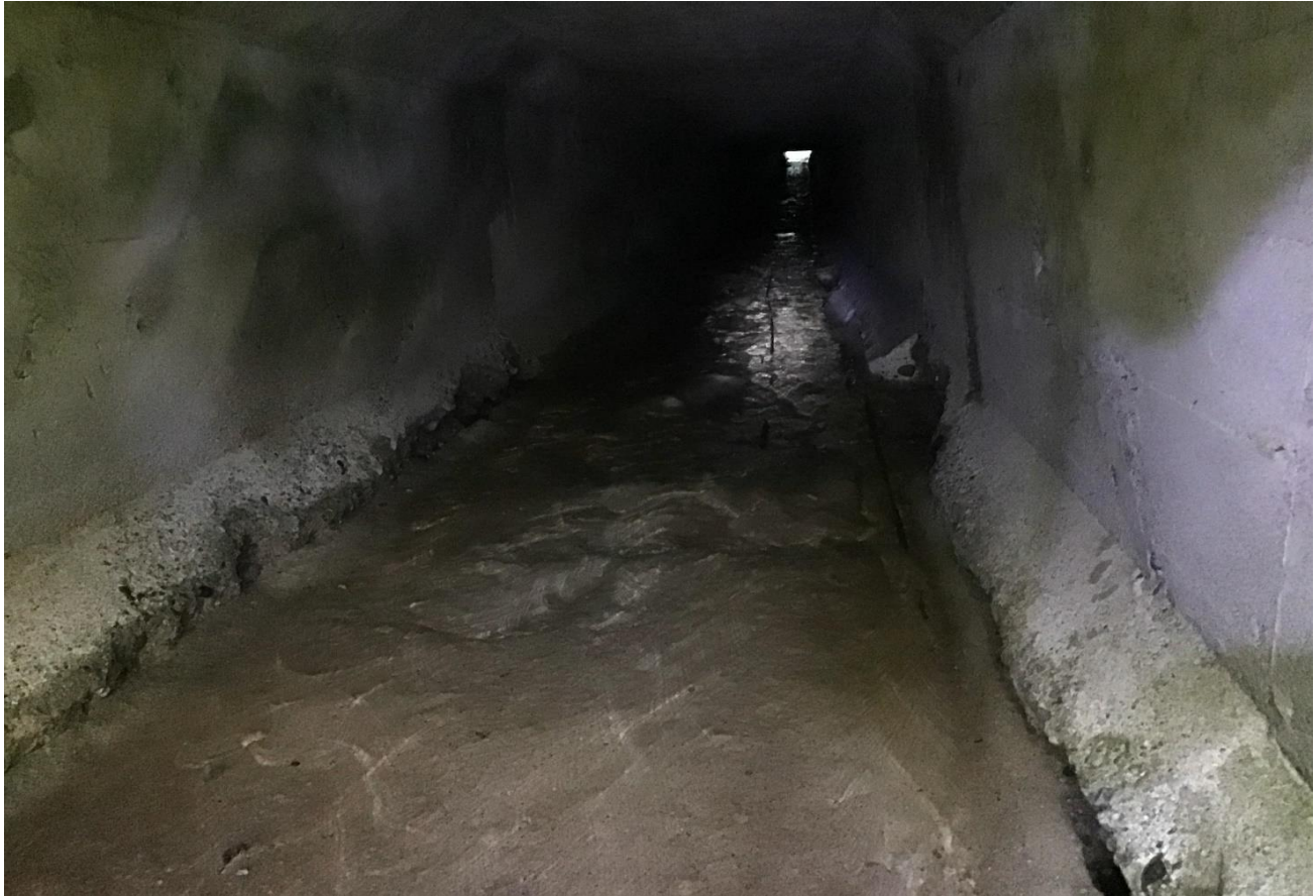
Channel floor scouring
